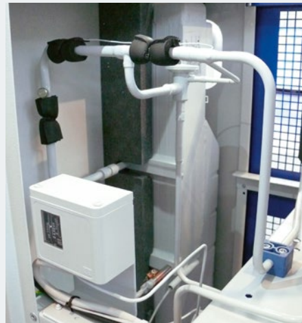
Inside of coated refrigeration dryer
